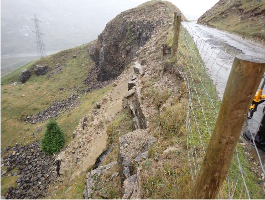
Plate 25: Chainage 228.0m to 250, Section of fence with no support due to crest failure
