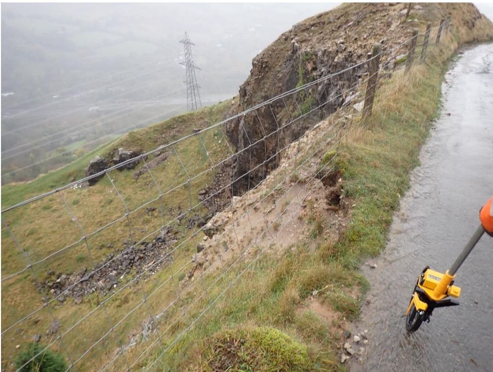
Plate 26: Chainage 243, Section of fence with no support due to crest failure with grip through verge.
