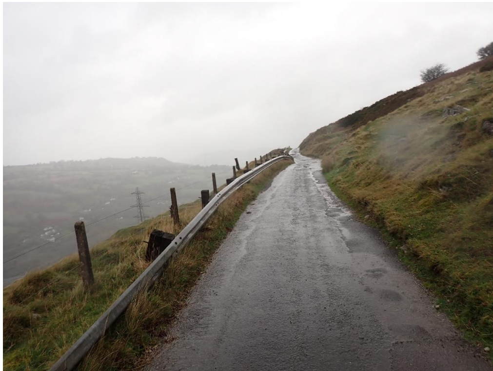
Plate 15: Chainage 104 to 112m, failed tilting VRS.
