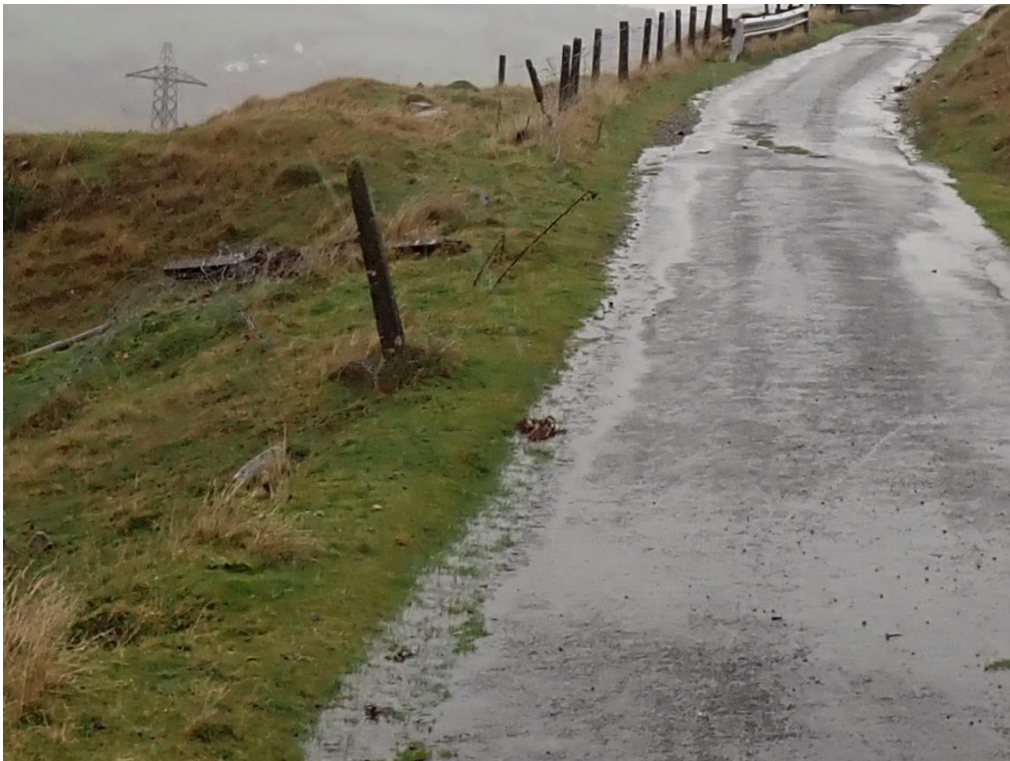
Plate 4 Chainage 32m. Local low point in carriageway - shallow grips in verge
