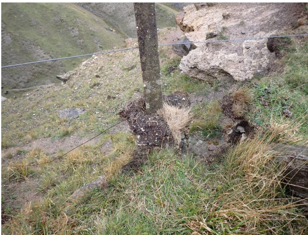
Plate 14: Chainage 100, failed fence post foundation.
