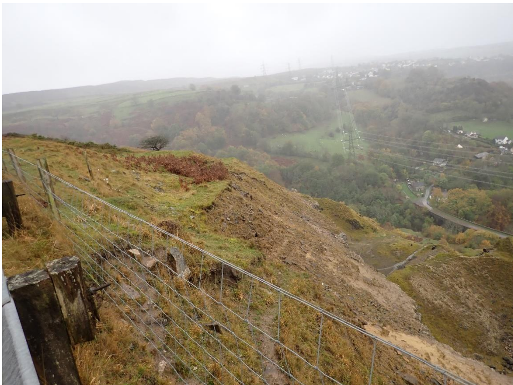
Plate 8: Chainage 69 to 79, The rock face / crest of slope moves within 0.5m of the back of the highway with surface slips on slope, leaning VRS, and stock fence with no supporting posts.
