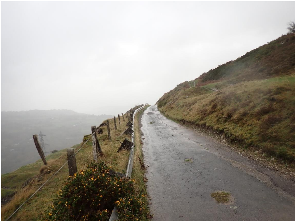
Plate 20: Chainage 150m, leaning VRS
