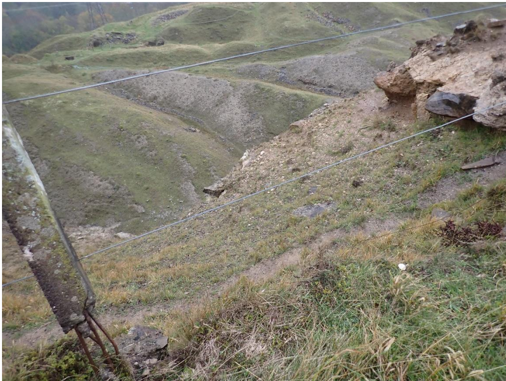
Plate 13: Chainage 97m, slip bowl below the road above quarry face with unsupported post
