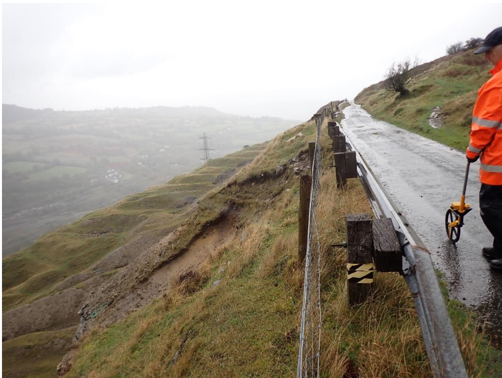
Plate 6: Chainage 69m The rock face / crest of slope moves within 0.5m of the back of the VRS
