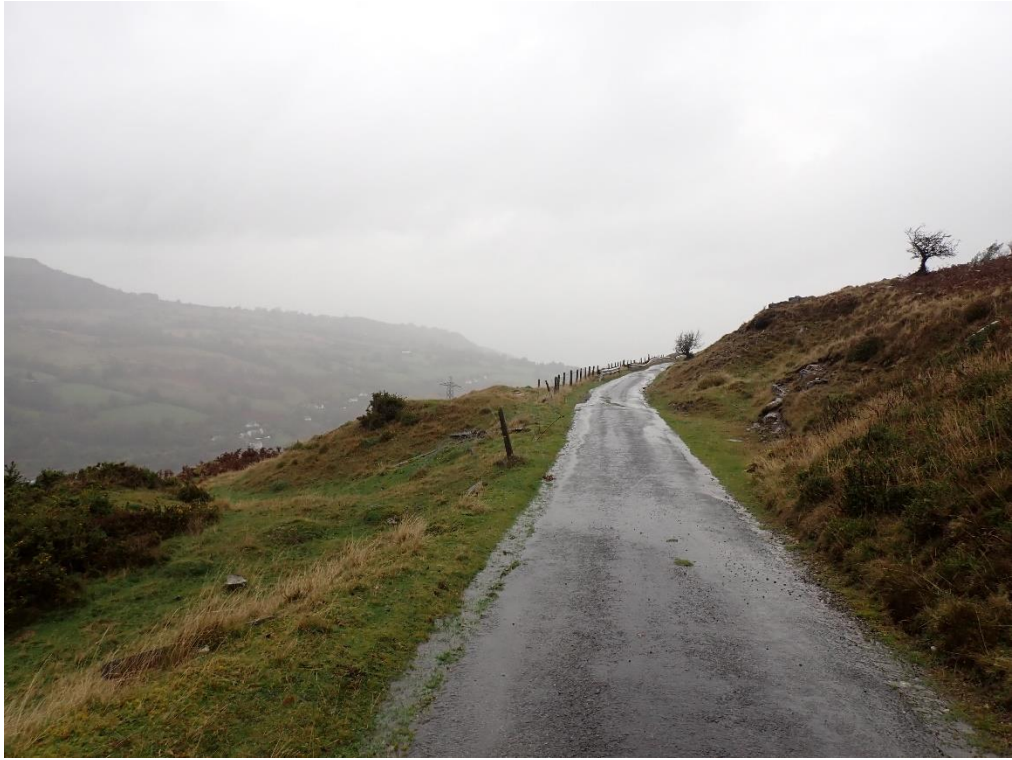
Plate 3 Chainage 32m. Local low point in carriageway - shallow grips in verge
