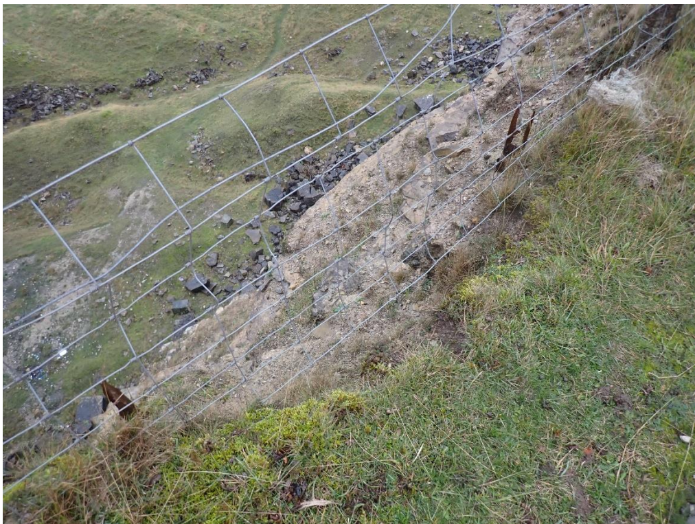
Plate 24: Chainage 215.0m, Section of fence with no support due to crest failure
