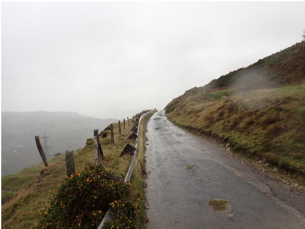
Plate 17: Chainage 141m, slip on slope below road close to carriageway. Note VRS leaning forwards
