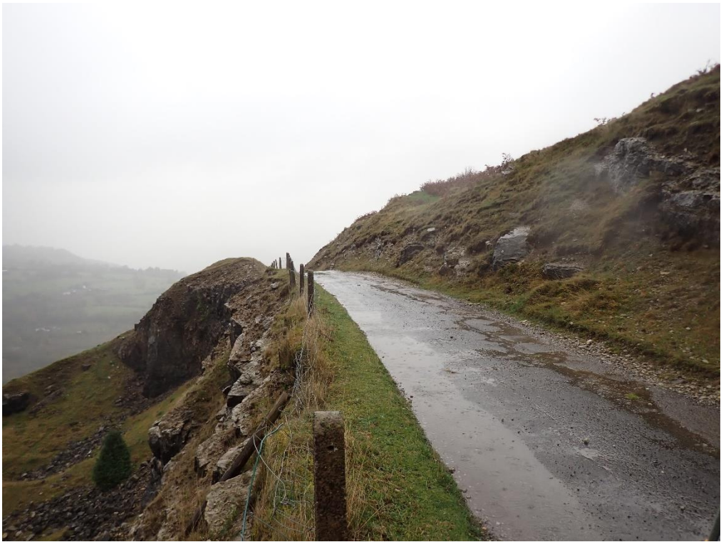
Plate 23: Chainage 202.0m, Failed section of fence
