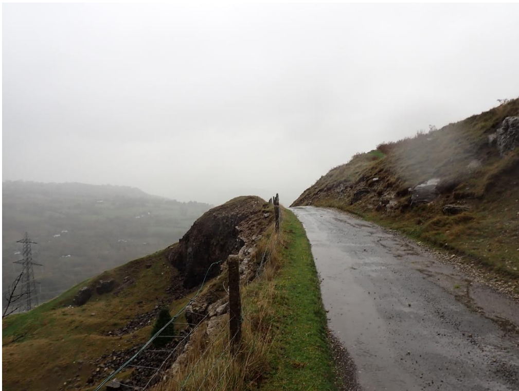
Plate 22: Chainage 199m, crest of slope / rock face close to edge of road. Note the poor quality of the fence.
